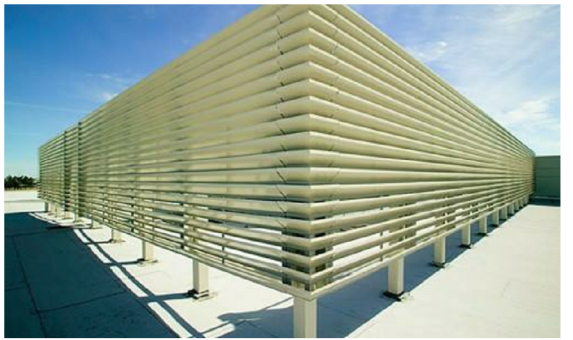
5. PENTHOUSE EQUIPMENT - SCREEN
